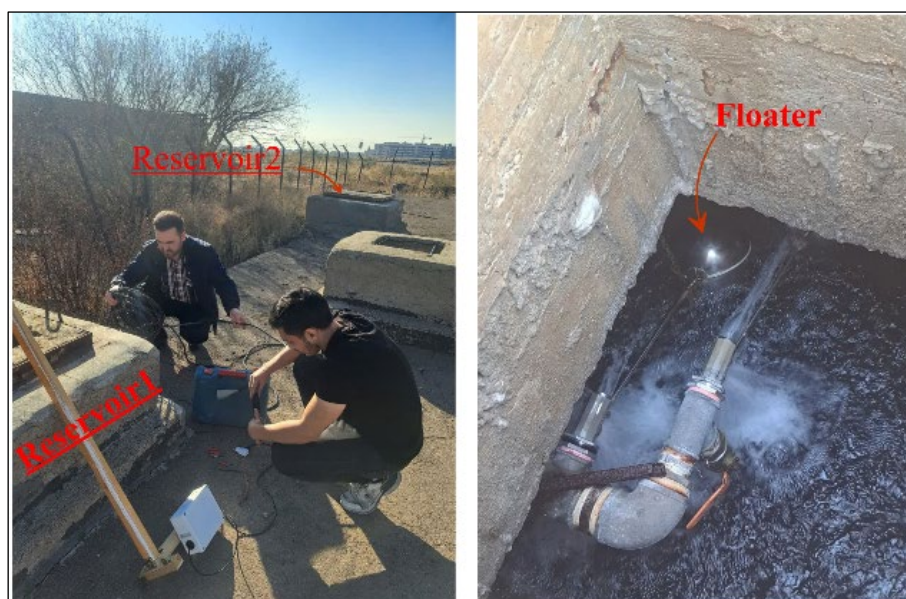
Fig. 5 View of the twin underground reservoirs supplying drinking water to Imam Khomeini International University
