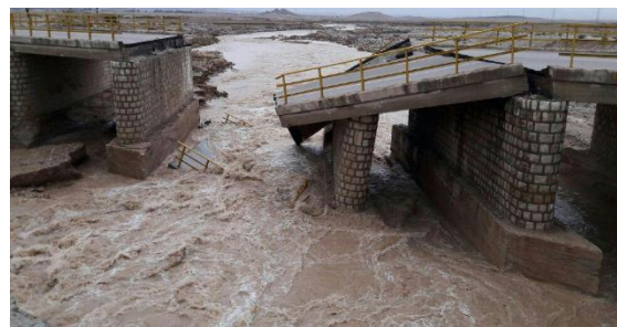
Fig. 1 A view of the destruction of the pier and bridge due to local scouring during the flood
