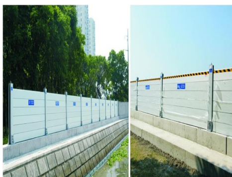
Fig 9 Precast flood wall to protect the study area
